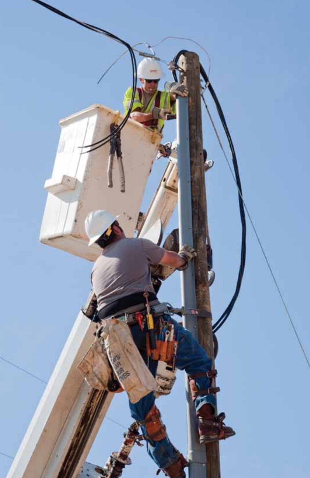
Nolin RECC line crews follow strict safety procedures to keep workers safe. Here, Josh Sanders on the pole and Nathan Yates in the bucket work on this de-energized line to prepare it for connection.
