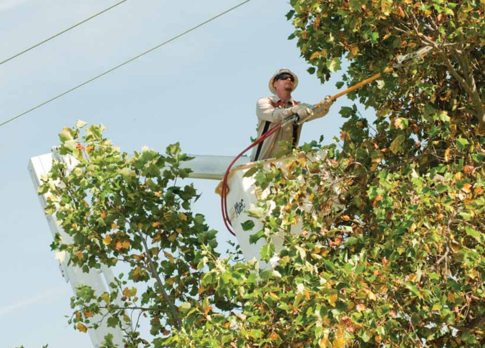
Keeping your electricity flowing means year-round trimming of vegetation that could damage power lines. Here, Robert Priddy, lead trimmer, uses a pole saw to remove threatening branches from Nolin RECC lines.
